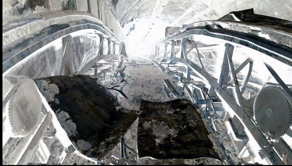
Charred remains of escalators at Euston Station after blast
